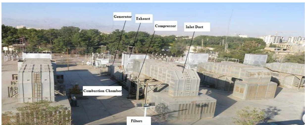
Figure 2 Case study power plant
